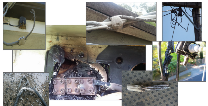
Supply service-line failures and degradation
